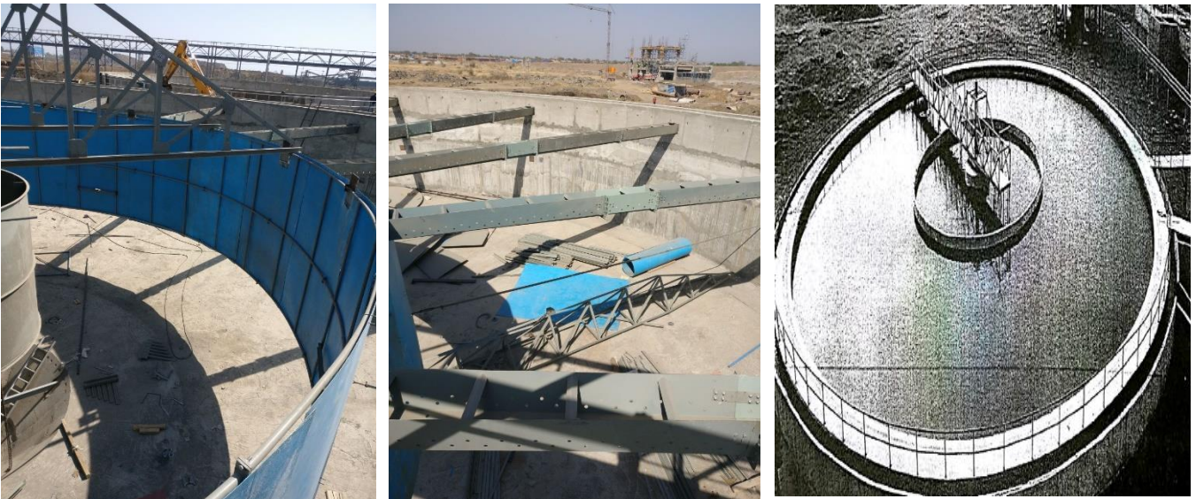
Fig 2.8: Onsite Pictures of clarifier at Malva II Plant.
